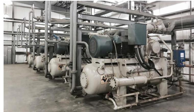
*Picture of RNG facility located at the Southern Landfill in Johnstown, PA
